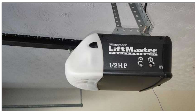
Chain drive opener noted.
