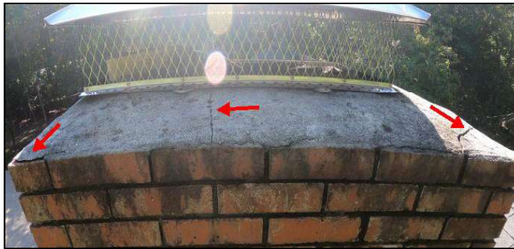
Chimney Mortar shows sign of deterioration. Recommend having repaired as necessary.
