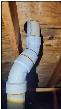
PVC plumbing vents
