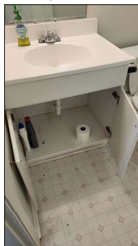
Appeared functional at time of inspection.
