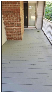
Appeared functional at time of inspection.
