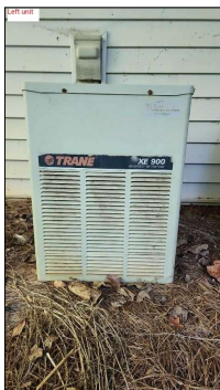
AC worked properly when tested during inspection.
