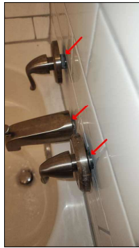
Tub faucet and fixtures are loose from the wall. Recommend securing properly to avoid water intrusion behind the fixtures.
