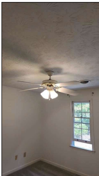
Operated normally when tested, at time of inspection.
