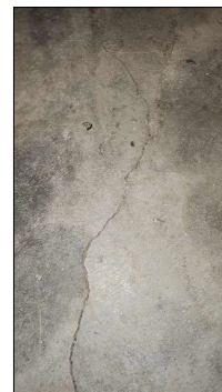
Common cracks noted.
