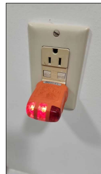
GFCI in place and operational
