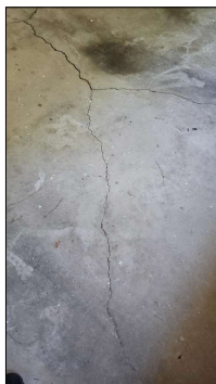
Common cracks noted.
