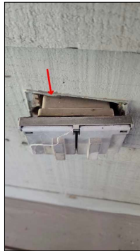
Exterior outlet is loose from wall at back deck.
