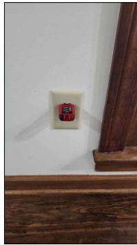
Outlets at living room windows did not function when tested. Recommend evaluation and corrections by a licensed electrician.
