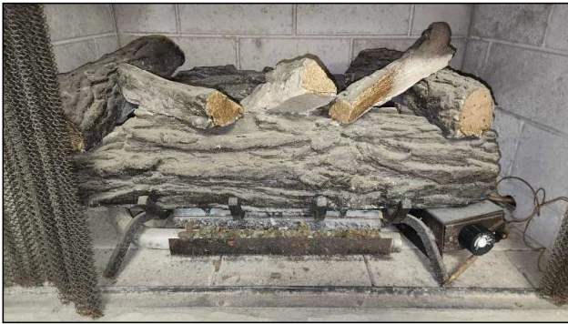
Gas Fireplace installed, but did not work when tested. Recommend having gas log specialist evaluate before closing.
