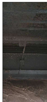
Damper in the open position.
