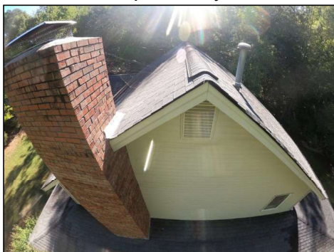
The roof is in fair condition and is beginning to show signs of wear. No major system safety or function concerns noted at time of inspection yet recommend evaluation by a licensed roofing contractor to assess roof life expectancy.
