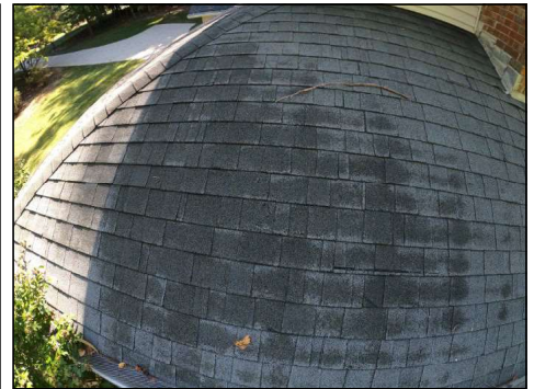
The roof is in fair condition and is beginning to show signs of wear. No major system safety or function concerns noted at time of inspection yet recommend evaluation by a licensed roofing contractor to assess roof life expectancy.
