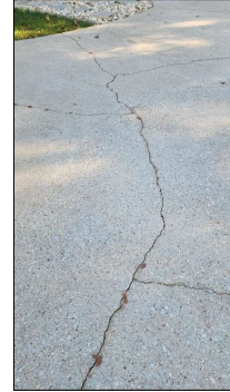
Common cracks noted.
