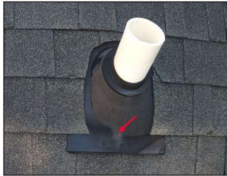
Shiners (exposed nail head) noted. This will rust and eventually cause a leak if not addressed.
