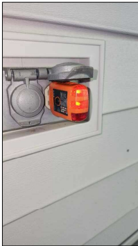
Outdoor receptacles at front of house are not GFCI protected, need to be updated.
