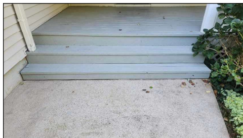
Appeared functional at time of inspection.
