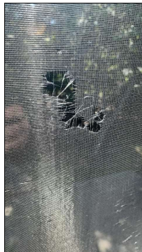
Some window screens damaged.
