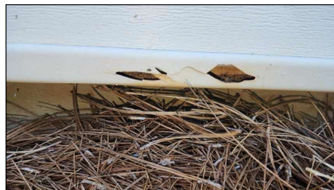
Some damaged areas noted.
