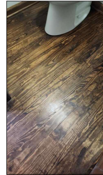
Bathroom floor appears to be in good/fair shape at time of inspection.
