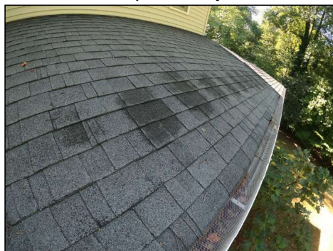
The roof is in fair condition and is beginning to show signs of wear. No major system safety or function concerns noted at time of inspection yet recommend evaluation by a licensed roofing contractor to assess roof life expectancy.
