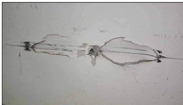
Damage to walls noted.
