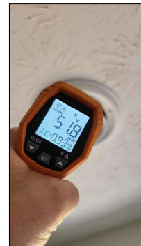
AC worked properly when tested during inspection.
