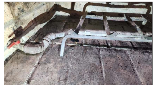
Gas log was not in place.
