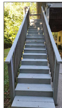
Appeared functional at time of inspection.
