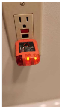
GFCI in place and operational
