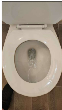
Observed as functional and in good visual condition.
