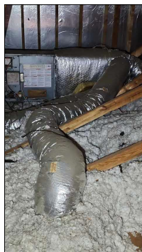
Ductwork appears functional.
