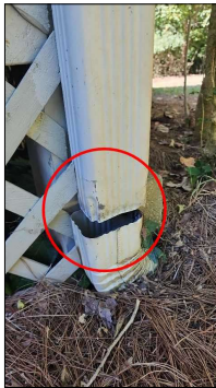
Downspout at front deck was not connected at time of inspection.
