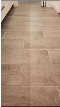
Bathroom floor appears to be in good/fair shape at time of inspection.
