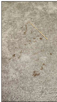
Carpet has stains in various places - recommend cleaning first, if not satisfied, change for new carpet or other flooring.
