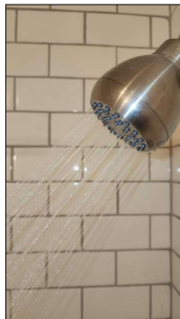
Worked properly during inspection.
