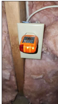
Outlets functioned properly when tested.
