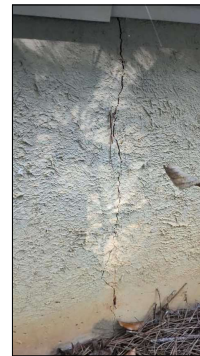
Normal cracks noted.
