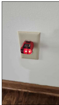
Outlet functioning properly.
