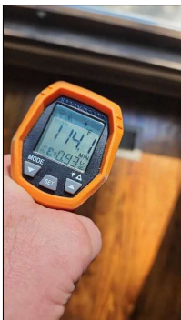
Heat functioning properly during inspection.
