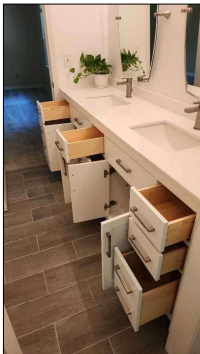
Appeared functional at time of inspection.
