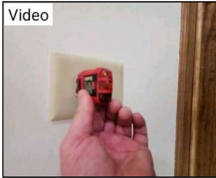
Outlet at living room wall is loose and tester lost function when juggled. Recommend evaluation and corrections by a licensed electrician.
