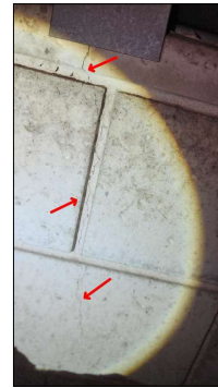
Cracks noted in the back of fireplace - recommend chimney sweep evaluate before using.
