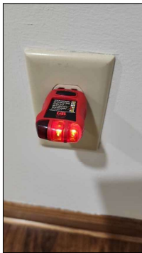
Outlet functioning properly.
