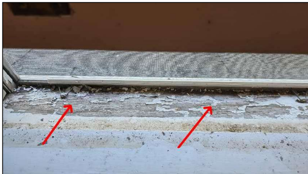
Some peeling paint at exterior sills noted.
