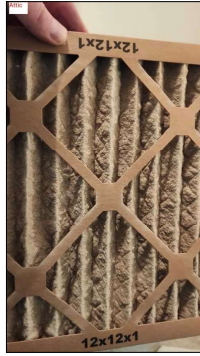
Furnace filter dirty. Needs replacement.
