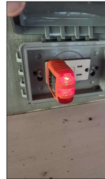
GFCI receptacles at back deck are in good condition and tested fine during inspection.
