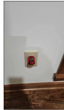
Outlets at living room windows did not function when tested. Recommend evaluation and corrections by a licensed electrician.
