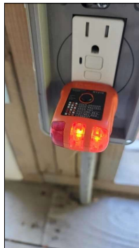
GFCI receptacles at back deck are in good condition and tested fine during inspection.
