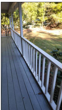
Appeared functional at time of inspection.
