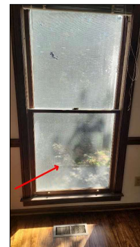
Window in kitchen dining area opens but will not stay up.
