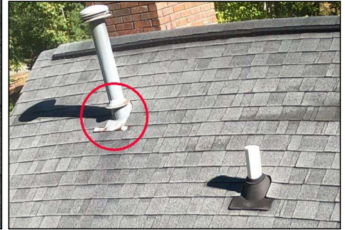
Vent bases are rusted, recommend replacement.
