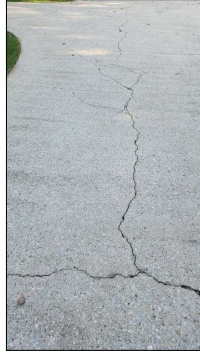
Common cracks noted.
