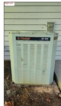
AC worked properly when tested during inspection.
