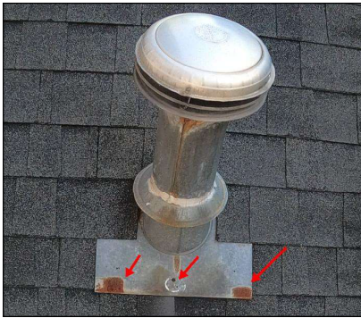
Vent bases are rusted, recommend replacement.
