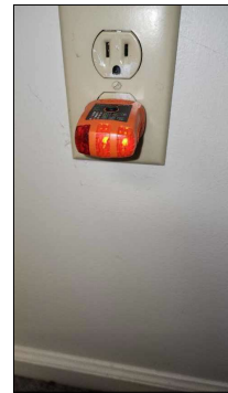
Outlet functioning properly.
