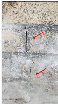
Cracks noted in the back of fireplace - recommend chimney sweep evaluate before using.
