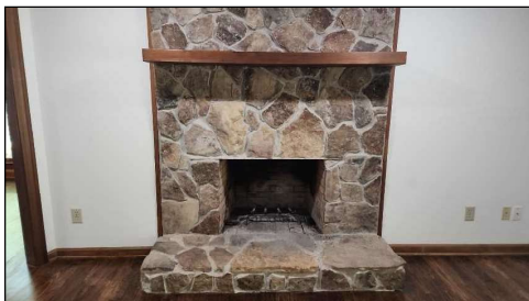
Fireplace was in fair condition.
