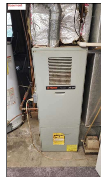
Heater looks fair and functioned properly at time of inspection.
