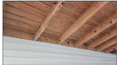
Appeared functional at time of inspection.
