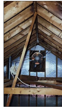
Thermostatically controlled Power Ventilator at gable vent noted.
