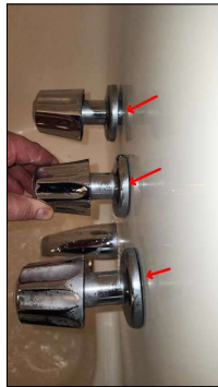
Tub faucet and fixtures are loose from the wall. Recommend securing properly to avoid water intrusion behind the fixtures.
