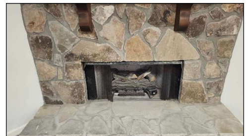
Fireplace was in fair condition.
