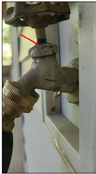
Spigot at back side of house leaks.
