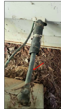
Missing/damaged insulation at A/C unit.
