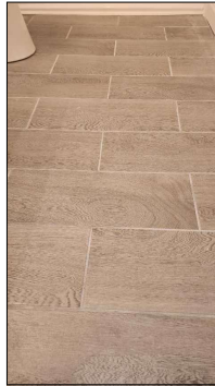
Bathroom floor appears to be in good/fair shape at time of inspection.
