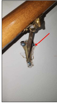
Handrail at stairs has a loose bottom bracket and some wall damage.
