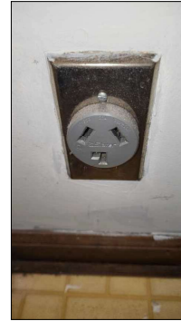
3 prong dryer outlet noted.
