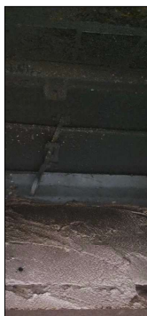
Damper in the closed position.
