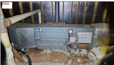
Heater looks fair and functioned properly at time of inspection.
