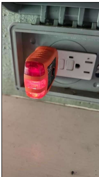
GFCI receptacles at back deck are in good condition and tested fine during inspection.
