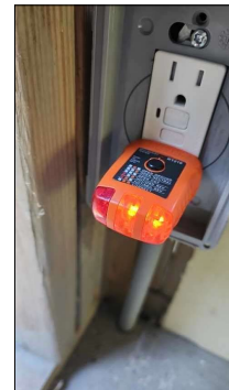
GFCI receptacles at back deck are in good condition and tested fine during inspection.
