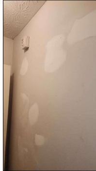
Some patched areas require sanding and painting.
