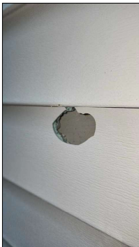
Some damaged areas noted.
