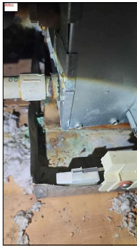
The heater base shows signs of rust from prior water intrusion.
