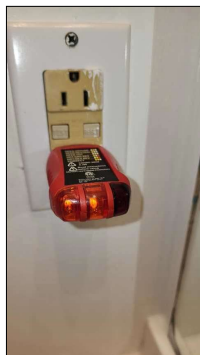
GFCI in place and operational
