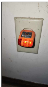
Outlets functioned properly when tested.
