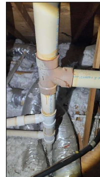
PVC plumbing vents
