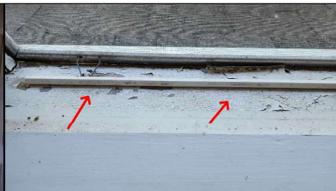
Some peeling paint at exterior sills noted.
