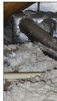
Ductwork appears functional.
