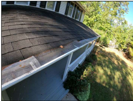
The roof is in fair condition and is beginning to show signs of wear. No major system safety or function concerns noted at time of inspection yet recommend evaluation by a licensed roofing contractor to assess roof life expectancy.
