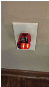
Outlet functioning properly.
