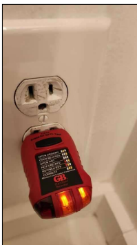
GFCI in place and operational
