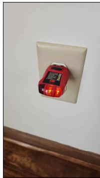
Outlet functioning properly.
