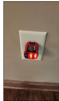
Outlet functioning properly.
