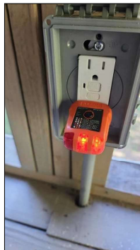
GFCI receptacles at back deck are in good condition and tested fine during inspection.
