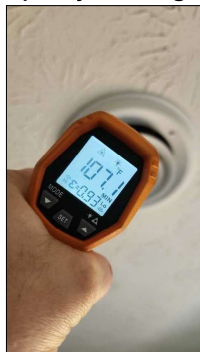
Heat functioning properly during inspection.
