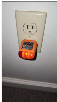
Outlet functioning properly.
