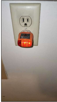
Outlet functioning properly.
