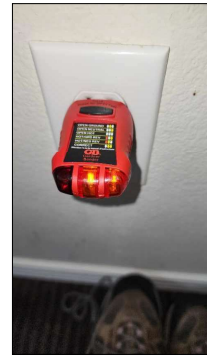
Outlet functioning properly.
