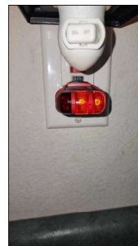
GFCI in place and operational.
