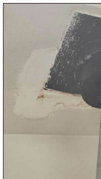
Some water damage at chimney box noted. Tested dry during inspection.
