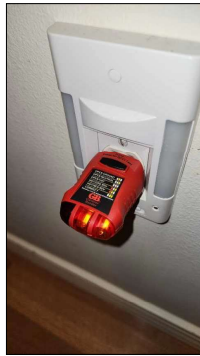
Outlet functioning properly.
