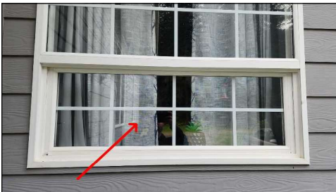
Some window screens missing.
