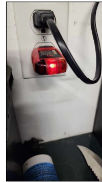
Open ground noted. Recommend corrections by a qualified electrician.
