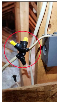
Connections made outside of a Junction Box, which is a potential shock or electrocution hazard.
