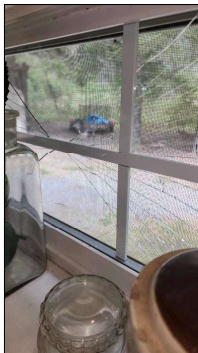
Broken/cracked glass pane in master noted, repairs needed.
