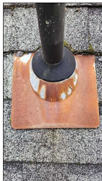
Vent bases are rusted, recommend replacement.
