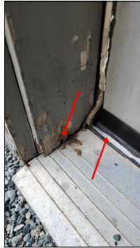
Garage access door threshold is loose at the base and door jamb is showing signs of degradation. Recommend corrections by a qualified carpenter.
