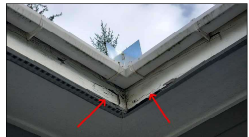
Some wood rot noted at fascia above garage access door. Recommend evaluation and corrections by a qualified carpenter.
