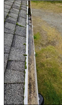
Ponding (sitting water) noted at gutter system. Need to change angle/slope to allow water to flow freely out of the gutter system.
