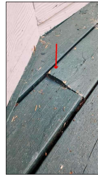
Warped deck board noted near bay window.
