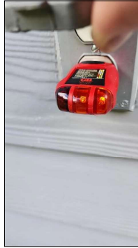
Outdoor receptacles are not GFCI protected, need to be updated.
