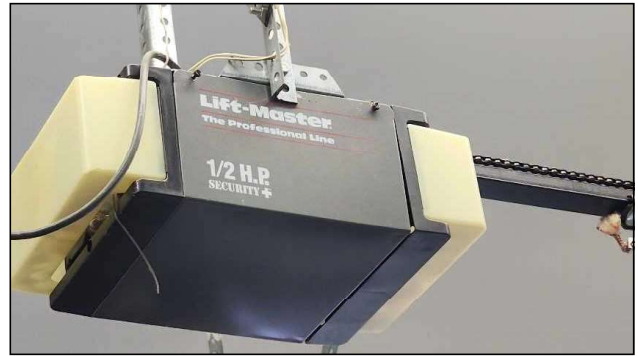
Garage door opener on left door was not functioning properly. Recommend servicing that door opener.
