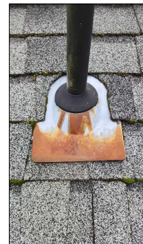
Vent bases are rusted, recommend replacement.
