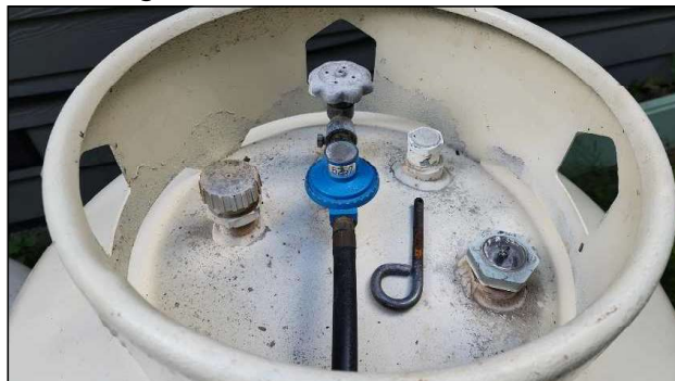
Meter located at exterior. All gas appliances have cut-off valves in line at each unit. No gas odors detected. No leaks noted when tested with meter.
