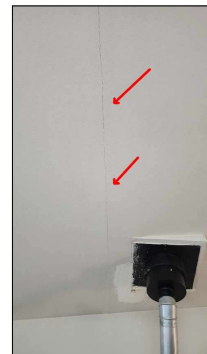
Seam cracks noted.
