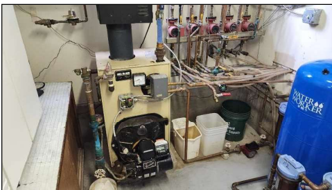
Boiler furnace for radiant floor heating noted. System operated properly during inspection. Recommend annual system service maintenance by a licensed plumber.
