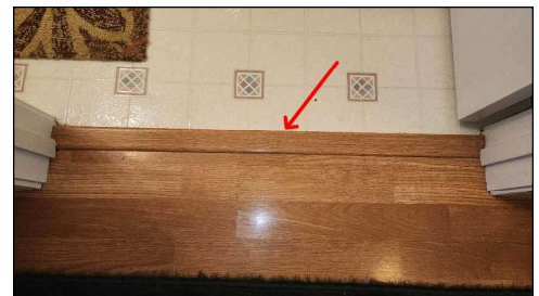
Transition in guest is loose and squeaky noted.
