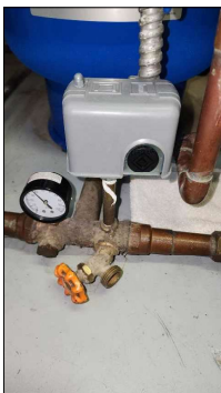
Pressure regulator noted.
