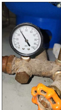
Pressure regulator noted.
