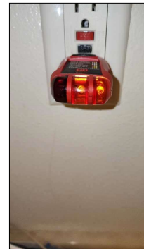
GFCI in place and operational
