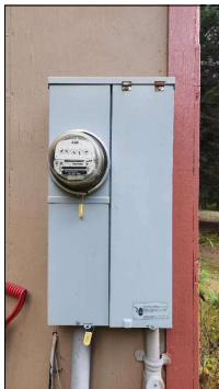
Main electric meter
