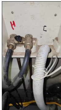
Appears to be functional.
