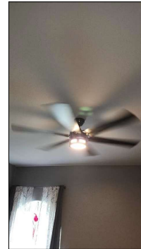
Operated normally when tested, at time of inspection.
