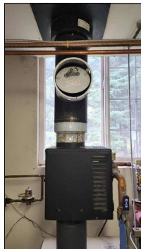
Boiler furnace for radiant floor heating noted. System operated properly during inspection. Recommend annual system service maintenance by a licensed plumber.
