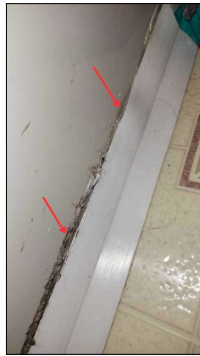
Cove base at guest bath is peeling away noted.
