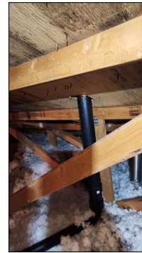
ABS plumbing vents
