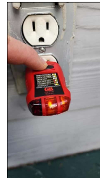
Outdoor receptacles are not GFCI protected, need to be updated.
