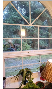
One or more window/s shows sign of loss of seal/condensation, recommend repair or replace to provide energy savings and prevent hazed window from limiting view out of window.
