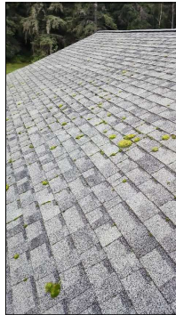
Moss on roof. This can lead to the premature failure of the roof and subsequent leaks. Recommend treating moss during its growing season (wet months) with a moss killer. For information on various moss treatment products and their pros and cons, visit http://bryophytes.science.oregonstate.edu/page24.htm .
