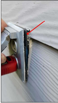
Outlet cover at garage wall is loose from receptacle noted.
