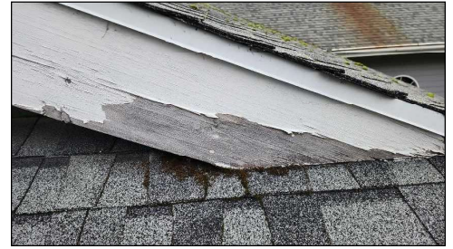
Peeling paint observed, suggest scraping and painting as necessary.
