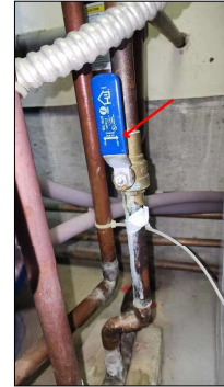
Main water cut off valve.
