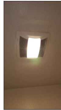
The bath fan was operated and no issues were found.
