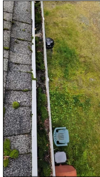
Clean gutters: Some/significant amounts of debris evident.
