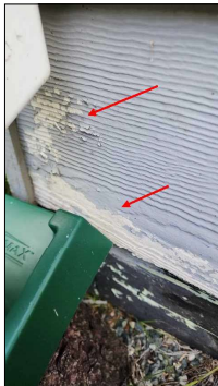
Some areas need restaining, or priming and repainting.
