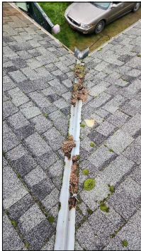
Clean roof areas: Significant amounts of organic debris evident.
