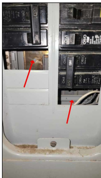
Open breaker panel slot(s) at panel box cover. Electrocutation hazard.
