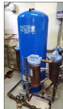
Pressure regulator noted.
