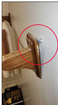
Towel bar loose from wall in master noted.
