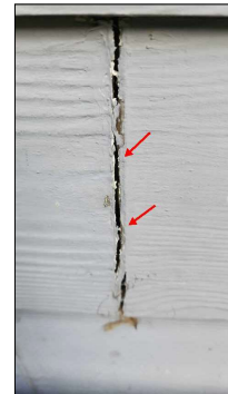
Recommend caulking and paint at some siding butt joint areas.
