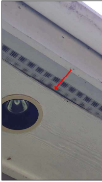
Soffit is coming loose in several areas around the perimeter of the house.
