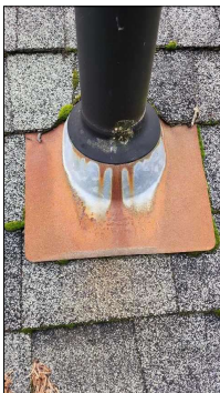
Vent bases are rusted, recommend replacement.
