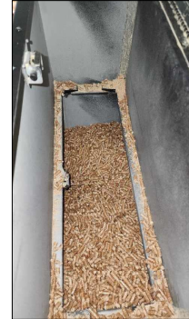
Pellet stove was in good condition and worked properly during inspection.
