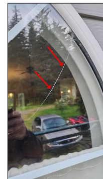
Window glass cracked.
