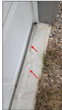
Common cracks noted.
