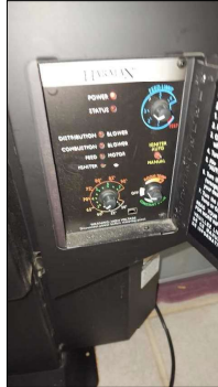
Pellet stove was in good condition and worked properly during inspection.
