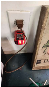
Outlets functioned properly when tested.
