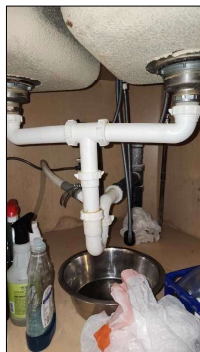
Plumbing looks to be in good condition. No apparent issues noted.
