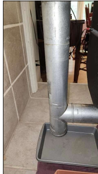
Pellet stove was in good condition and worked properly during inspection.
