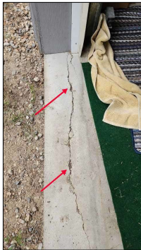
Common cracks noted.
