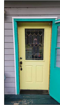
Front door looks to be in good condition and worked properly during inspection.
