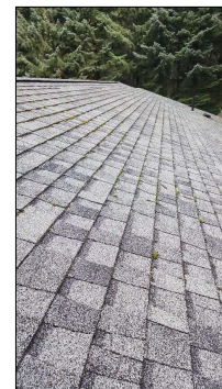
Roof is beginning to show significant signs of wear. Recommend evaluation by a licensed roofing contractor to determine life of roof and/or price quote for replacement.
