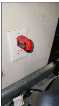
GFCI in place and operational.
