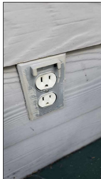
Waterproof receptacle cover missing noted.
