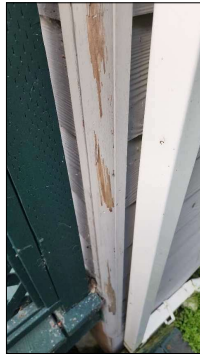
Peeling paint noted.
