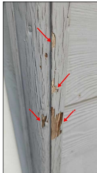
Some areas need restaining, or priming and repainting.
