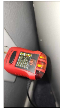
Outlet working during inspection.
