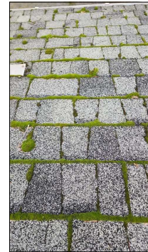
Moss on roof. This can lead to the premature failure of the roof and subsequent leaks. Recommend treating moss during its growing season (wet months) with a moss killer. For information on various moss treatment products and their pros and cons, visit http://bryophytes.science.oregonstate.edu/page24.htm .
