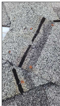
Rusted nailheads showing. These may leak at any time. Recommend caulking nailheads.
