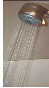
Worked properly during inspection.
