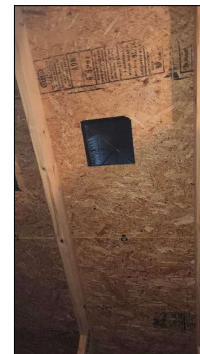
Fixed, roof-field exhaust vent noted.
