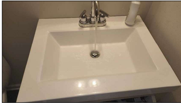
Operated normally, at time of inspection.
