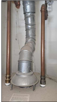
No major deficiencies observed at the visible portions of the supply piping.
