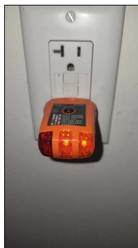
Outlets functioned properly when tested.
