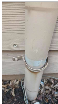
Bracket is loose from wall at service conduit noted.
