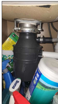
Operated - appeared functional at time of inspection.
