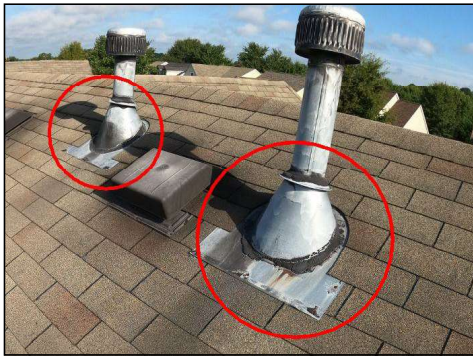
Vent bases are rusted and caulking looks to be degrading, recommend replacement.
