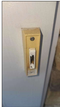
Door bell cover is broken noted.
