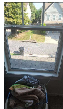
Window in master bedroom will open but not stay up noted.
