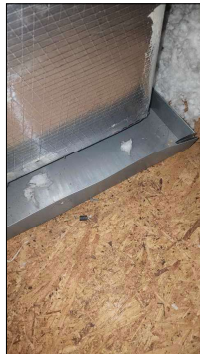
The heater base appears to be functional.
