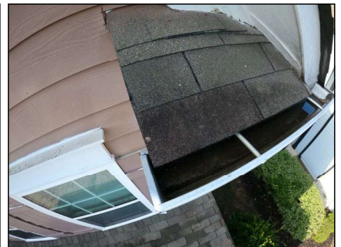
Ponding (sitting water) noted at gutter system. Need to change angle/slope to allow water to flow freely out of the gutter system.
