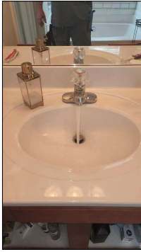
Operated normally, at time of inspection.
