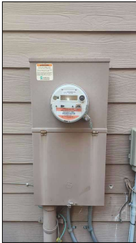
Main electric meter
