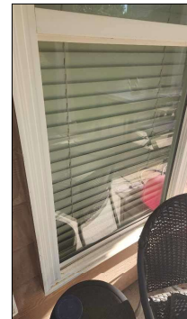
Some window screens missing and some damaged.
