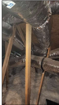
Ductwork appears functional.
