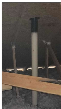
PVC plumbing vents
