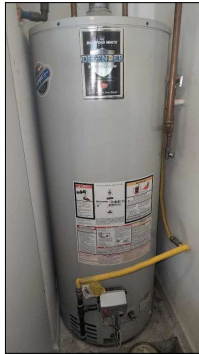
The water heater enclosure is functional.
