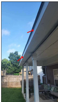
Recommend installing gutters at back patio roof.
