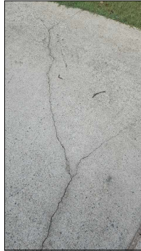
Common cracks noted.
