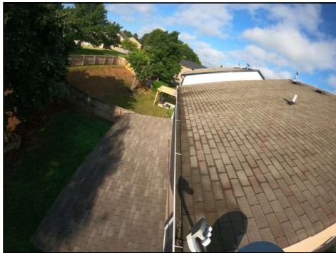
Roof looks to be original, is showing some signs of degradation and may need to be replaced in the near future. Recommend evaluation for life expectancy and price quote for replacement by a licensed roofing contractor.
