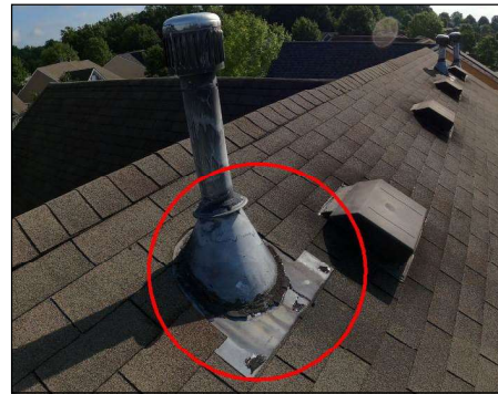
Vent bases are rusted and caulking looks to be degrading, recommend replacement.
