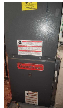
Heater looks good and functioned at time of inspection.
