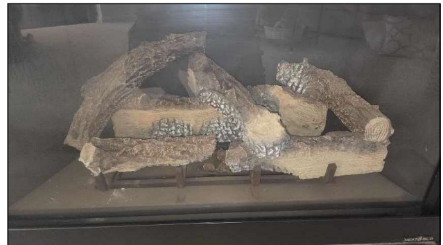
Gas Fireplace installed, but did not work when tested. Recommend having gas log specialist evaluate before closing.
