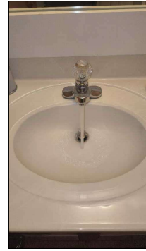
Operated normally, at time of inspection.
