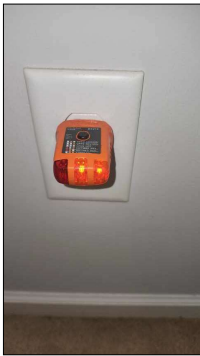
Outlet functioning properly.
