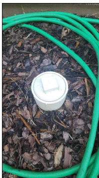
Drain pipe clean out noted.
