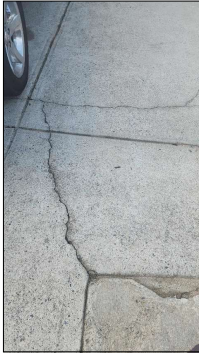
Common cracks noted.
