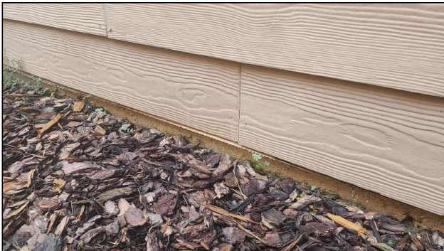
No deficiencies were observed at the visible portions of the structural components of the home.
