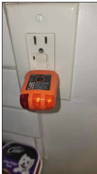
GFCI in place and operational.
