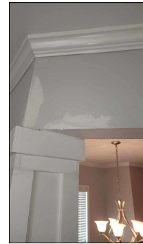
Some areas have patchwork noted.
