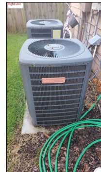
AC unit functioned during inspection
