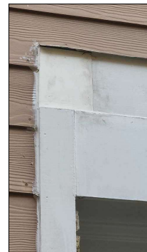
Evidence of repairs observed, unable to determine the effectiveness of these repairs.
