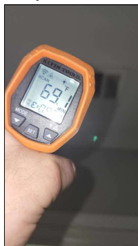
AC at main did not reach temps I was looking for - recommend HVAC specialist to evaluate to see if it needs freon or has other issue.
