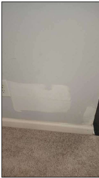
Some areas have patchwork noted.
