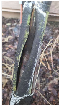
Missing/damaged insulation at A/C unit.
