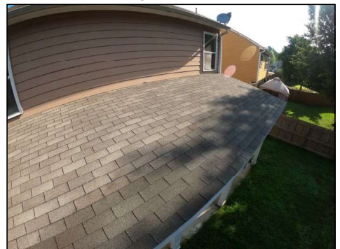
Roof looks to be original, is showing some signs of degradation and may need to be replaced in the near future. Recommend evaluation for life expectancy and price quote for replacement by a licensed roofing contractor.
