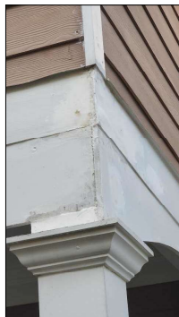
Evidence of repairs observed, unable to determine the effectiveness of these repairs.
