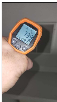
Differential temps at main floor return were not within the accepted range of 13 to 20 degrees, recommend HVAC specialist to give professional opinion on issue.
