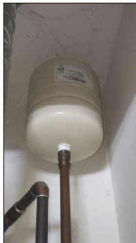
Expansion tank is in place and appears functional.
