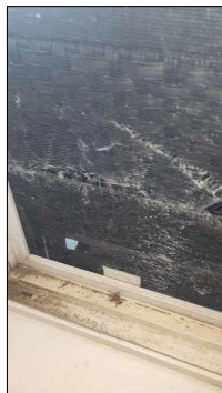
Some window screens missing and some damaged.
