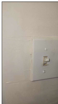
Some areas have patchwork noted.
