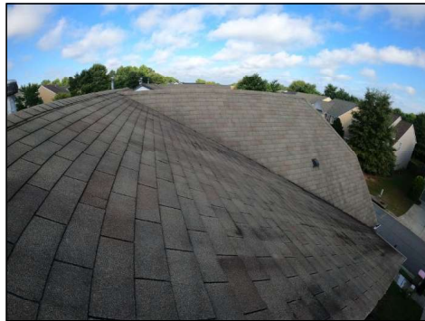
Roof looks to be original, is showing some signs of degradation and may need to be replaced in the near future. Recommend evaluation for life expectancy and price quote for replacement by a licensed roofing contractor.
