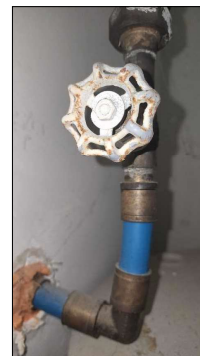
Main water cut off valve.
