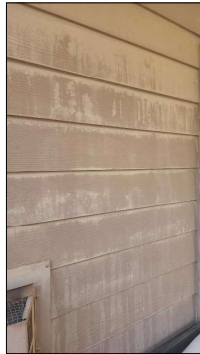
Recommend painting maintenance at some areas.
