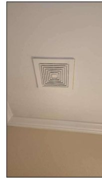
The bath fan was operated and no issues were found.
