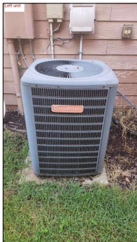
AC unit functioned during inspection
