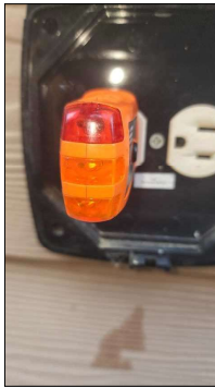
GFCI receptacles are in good condition and tested fine during inspection.
