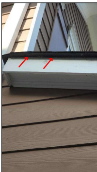
No drip edge noted at eaves.
