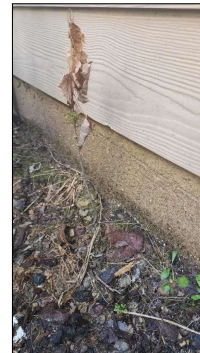
No deficiencies were observed at the visible portions of the structural components of the home.
