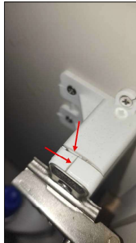
Cabinet hinges in half bath are cracked noted.
