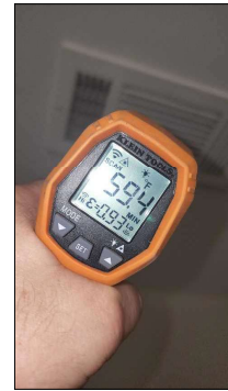
AC worked properly when tested during inspection.
