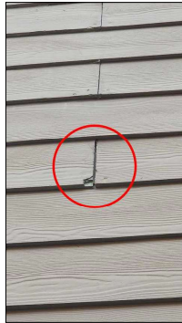
Some damage noted.
