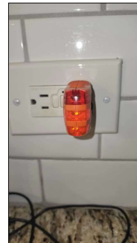
GFCI in place and operational.
