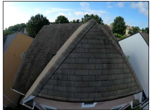
Roof looks to be original, is showing some signs of degradation and may need to be replaced in the near future. Recommend evaluation for life expectancy and price quote for replacement by a licensed roofing contractor.
