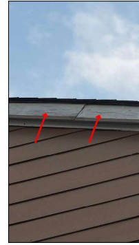
Peeling paint at barge rafters noted.
