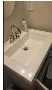
Composite tops noted.
