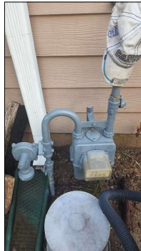
Meter located at exterior. All gas appliances have cut-off valves in line at each unit. No gas odors detected. No leaks noted when tested with meter.
