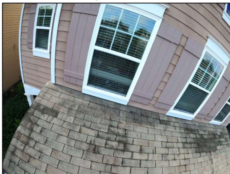
Roof looks to be original, is showing some signs of degradation and may need to be replaced in the near future. Recommend evaluation for life expectancy and price quote for replacement by a licensed roofing contractor.
