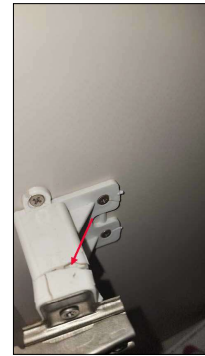
Cabinet hinges in half bath are cracked noted.
