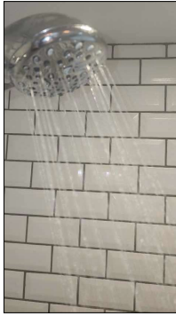
Worked properly during inspection.
