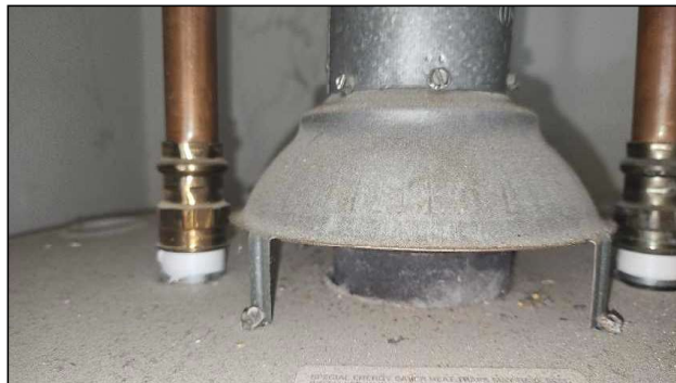
The vent appears to be installed/mounted correctly.
